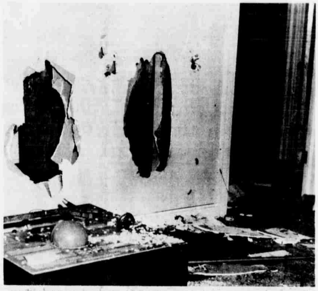
VANDALS AT WORK -- Two young Littlefield boys admitted destruction to a house occupied by Kenneth Seals on West 1st. Above is the living room of the home as found by firemen summoned to the home to extinguish a fire Sunday afternoon. In the picture are the large holes knocked in the walls between the living room and bedroom, a television set over turned and on the back on the tv set a broken jar of vegetables.
