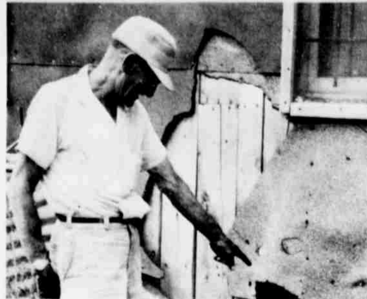
CITY EMPLOYEE CLAUD GRIMES POINTS TO HOLE... where city warehouse was burglarized Monday night of a quantity of confiscated liquor. (Staff Photo)
