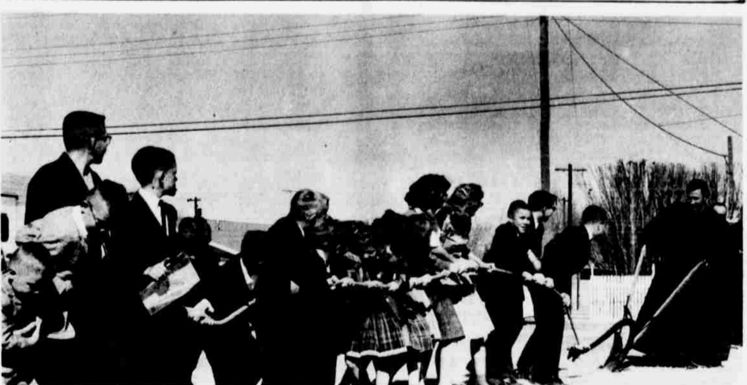
EMMANUEL LUTHERAN CHILDREN played a big part in the official ground breaking ceremonies for a new $60,000 sanctuary Sunday morning. Here they are shown pulling a breaking plow with the Rev. E. M. Hohle guiding the plow. When they all pulled together, they plowed a nice furrow through the heavy bermuda grass.
