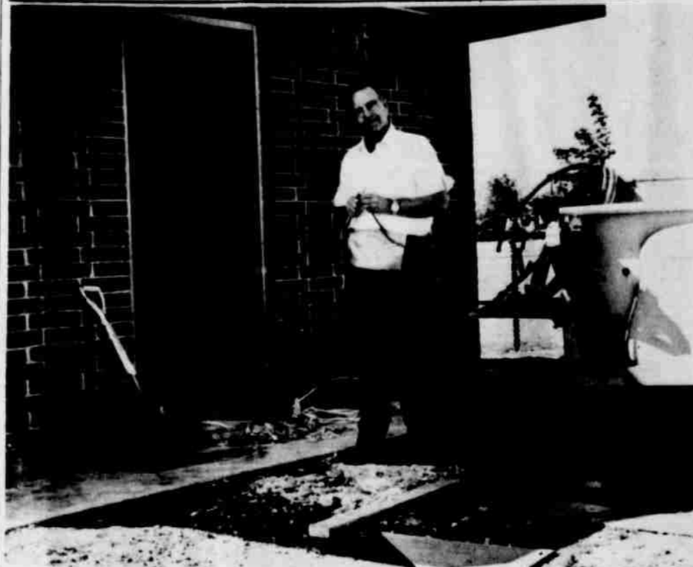
CHARLES DUVAL, chairman of the park committee for Rotary, pauses for a moment in his construction of a brick building in Crescent Park, sponsored by Rotary, which will
