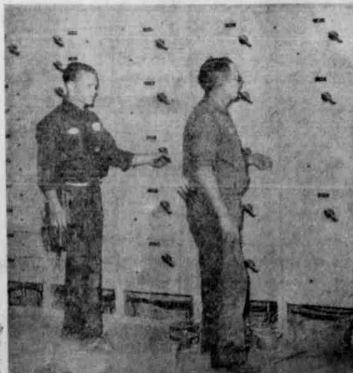
This huge display of electrical breaker and control switches keeps tab on the 30 electrical motors which power the different facilities in this modern new gin.
