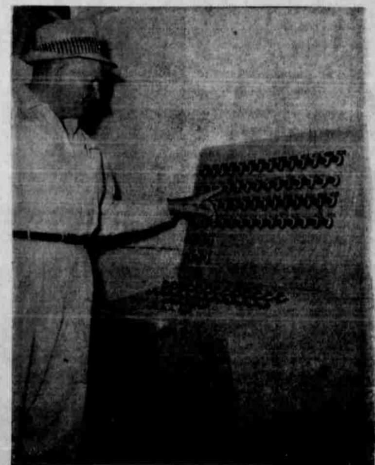
Gin manager Rex Love looks over the push button control panel which maintains touch contact with all of the gin's operations. No more risking catching hands in gin stands with this new electrical innovation.
