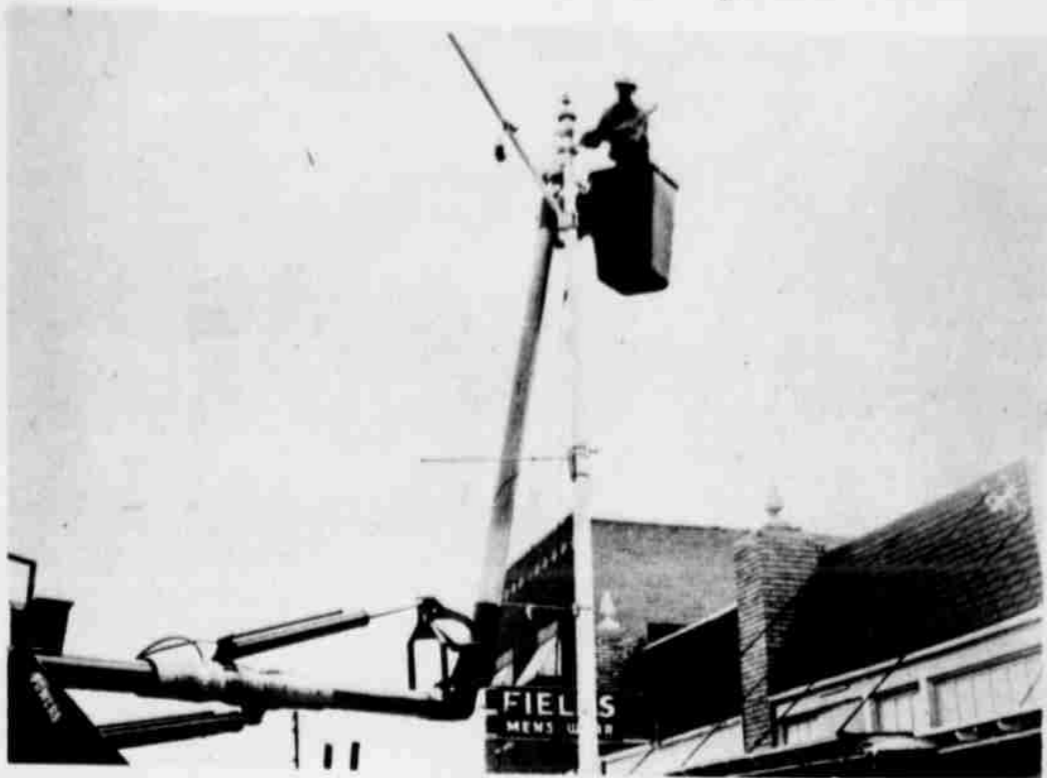
UP IN THE AIR -- Southwestern Public Service employees spent a good deal of time up in the air during the construction portion of the downtown project as they installed new 54,000 lumen mercury vapor lights on Phelps Ave. and new 20,000 lumen lights on the side streets and on XIT and LFD. They also worked in conjunction with General Telephone to erect new poles on XIT and LFD. ---NEWS STAFF PHOTO
