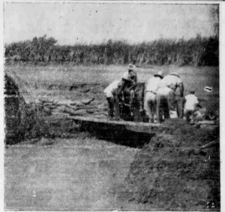
CANAL BROKEN —A break in the Mercedes irrigation district main canal left the south Texas city without water. Above, workmen rush to repair the break in the canal bank. Emergency water supplies were trucked to Mercedes. Fishermen had a holiday harvesting stranded gar and catfish with pitchforks and machetes. —AP Photo
