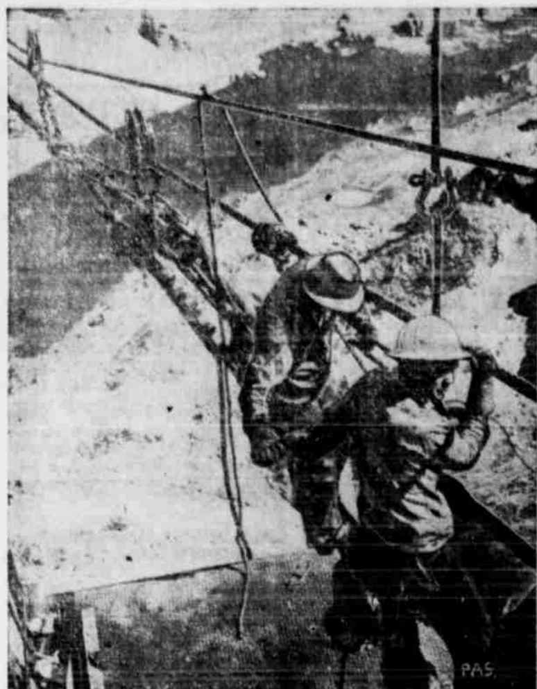
REDDING, Cal. . . . Seven hundred feet above the Sacramento river, these workers are stringing wires for the 460 foot cableway from the head tower at the Shasta Dam. Destined to be the world's second largest concrete dam, it will be used for multiple conservation purposes in the great Central Valley of California.
