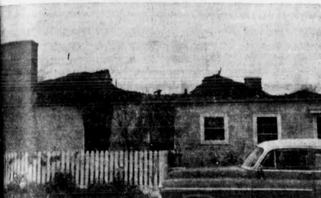
THE GAPING HOLE in the roof of the J. D. Hagler residence, 1223 S. Phelps, stands in mute testimony of a disastrous blaze which gutted the interior Monday morning causing damage estimated at $20,000 to $25,000.
