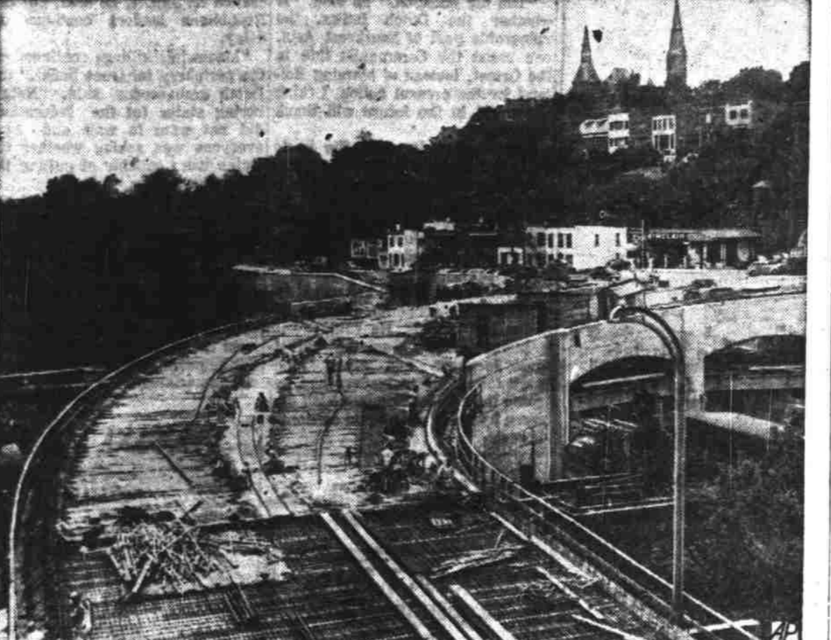
ELEVATED HIGHWAY — Workmen prepare to pave Washington's first elevated highway, Whitehurst Freeway, which will eliminate a traffic bottleneck by bypassing Georgetown and cobbled-up M Street. On hill are George Washington University buildings.
