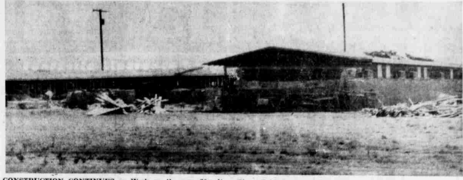
CONSTRUCTION CONTINUES — Work on the new 20-unit Crescent Park Motel continued in full swing this week despite soaring temperatures. Owners of the new motel, Ace Bridwell and Buck Oldham, hope to have all work completed by Sept. 1.
