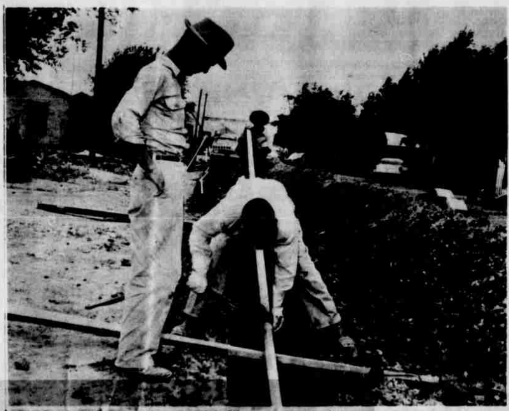
ON THE LINE—Water facilities to Littlefield's "flats" area are being improved with the installation of new lines on several streets and the lowering of old lines on others. The
