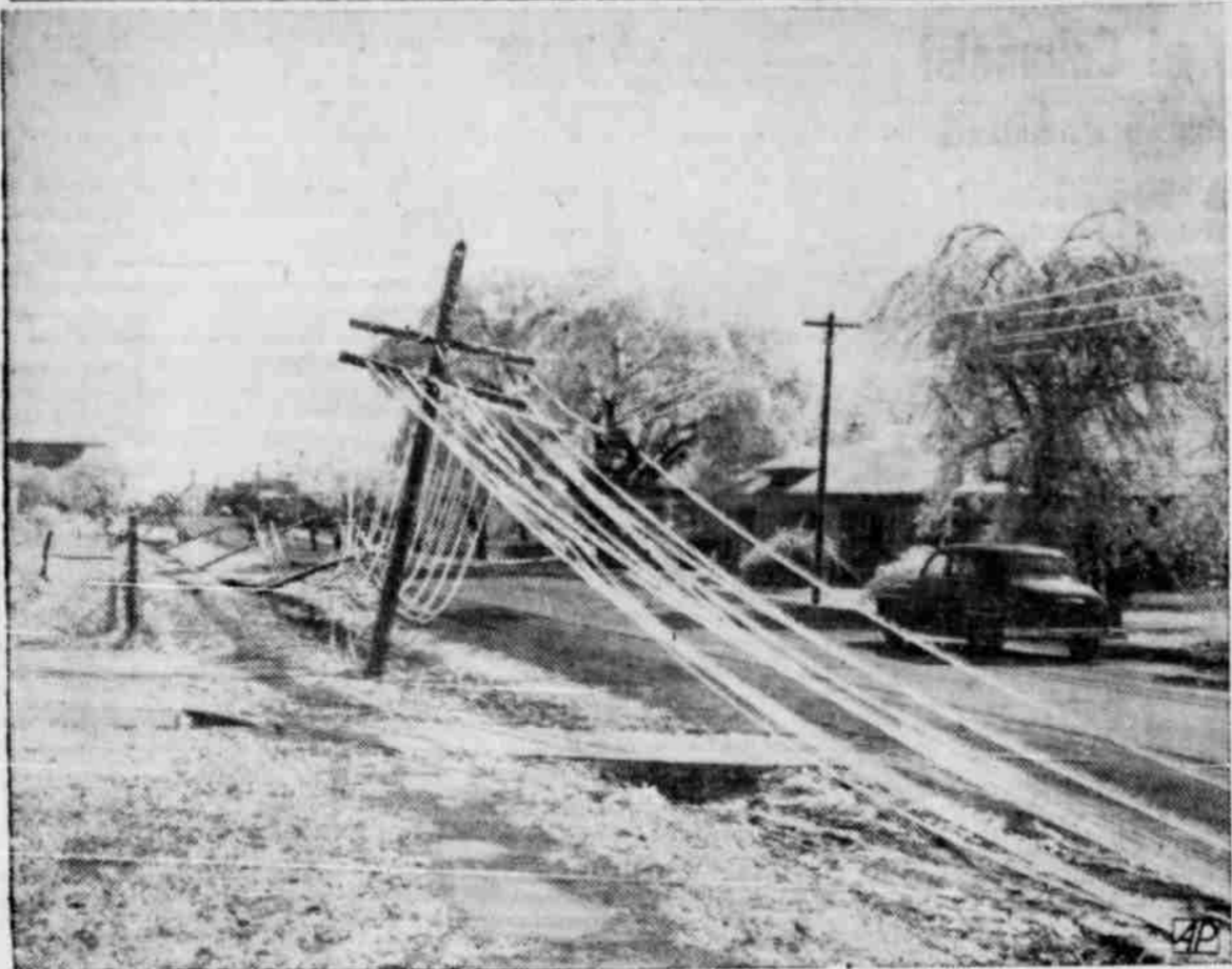
ICE DOWNS WIRES —Freezing rain caused much damage in North and East Texas during a storm that swept the state in the second week in February. Line crews had plenty of work repairing damaged lines like those at Cumby, Tex. Snow, sleet and ice melted rapidly and helped relieve a drought condition. (AP Photo)
