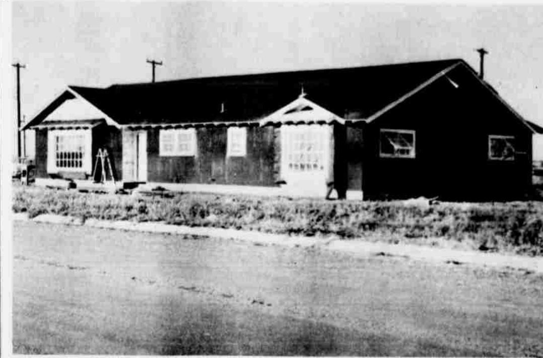
CONSTRUCTION CONTINUES ON BOOM -- Shown above is just one of the new homes and other building begun during September. City building permits for this year topped the million dollar mark for the year and are out in front of the record year. (Staff Photo)
