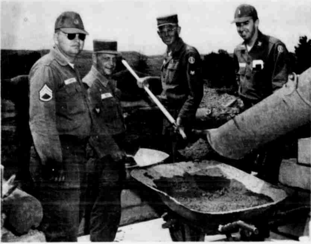
TEXAS RESERVISTS are busy at pouring concrete at one of Fort Carson's hand grenade ranges. While in Colorado for their annual summer camp training from Company B of the 980th Engineer Battalion these citizen-soldiers assisted with many such construction projects. Shown here from the left is Sargent Melvin Campbell of Littlefield along with Sp/4 Henry Poff, Sp/4 Jim Woodell, and 1/Lt. Robert R. Cochrane of Lubbock. They returned home June 20th by aircraft of the Air National Guard.
