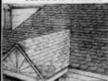
Damage to wallpaper, furniture, and walls is expensive. It's cheaper to re-roof.
