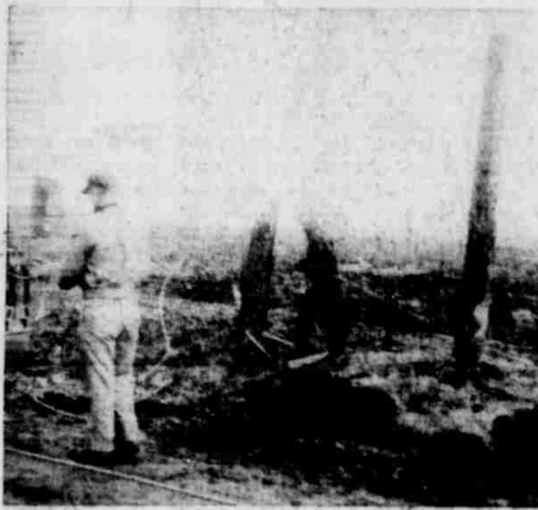
QUEER HAPPENINGS — Shown above are Max Wingham and Charles Smith of the Southwestern Public Service repairing lines in front of the J. E. Padon. Two poles are shown side by side with one standing unhurt and other broken into and lying in the field beyond. There were two separate instances of this, less than 50 yards apart. (Staff Photo)
