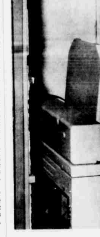
EXPLOSION RIPS OUT WALL--An explosion in a washing machine at the home of Clyde Wood at 500 W. 4th late Monday afternoon did extensive damage to the inside of the home near the machine. A door was blown off and in half striking Mrs. Wood and injuring her. The wall behind the washer (shown above) was knocked out. Littlefield volunteer firemen answered the call but there was no fire. (Staff Photo)
