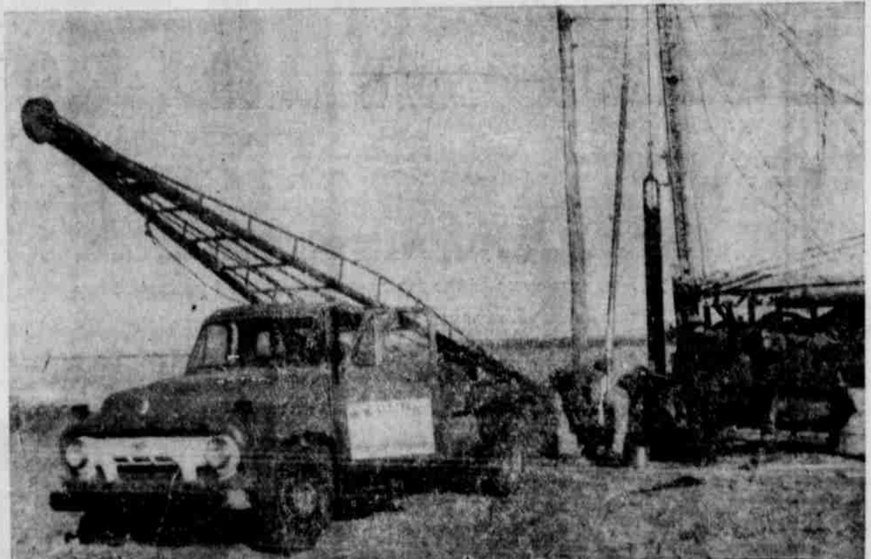
PICTURED ABOVE IS ONE OF THE W-W ELECTRIC DRILLING RIGS in operation. The local firm has an established reputation of fair dealing in both the sale and installation of pumps.
