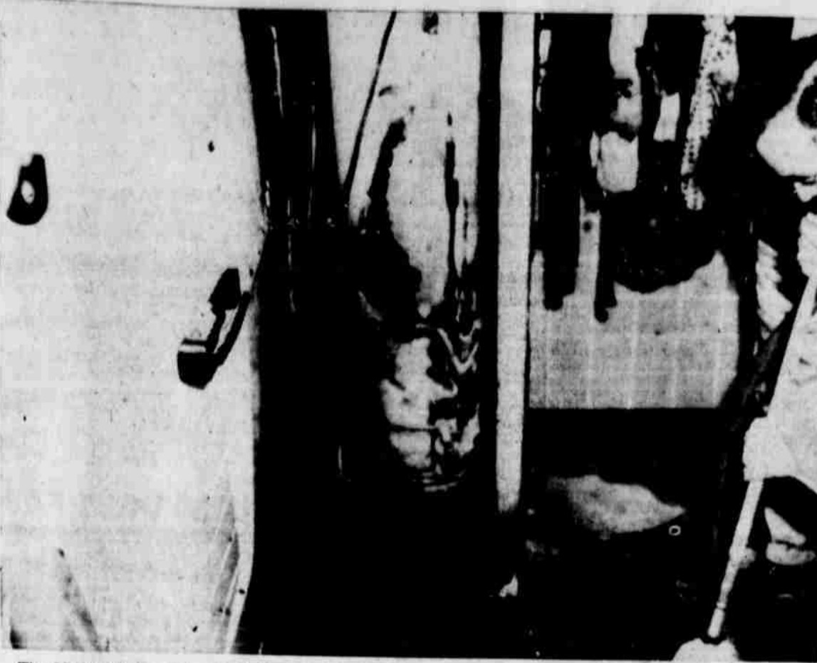
The McAmish home in the College Heights Addition was badly damaged in a fire at 6:30 p. m. Sunday. The clothing, refrigerator and deep freeze was a total loss. A defective water heater started the fire. (Staff Photo)
