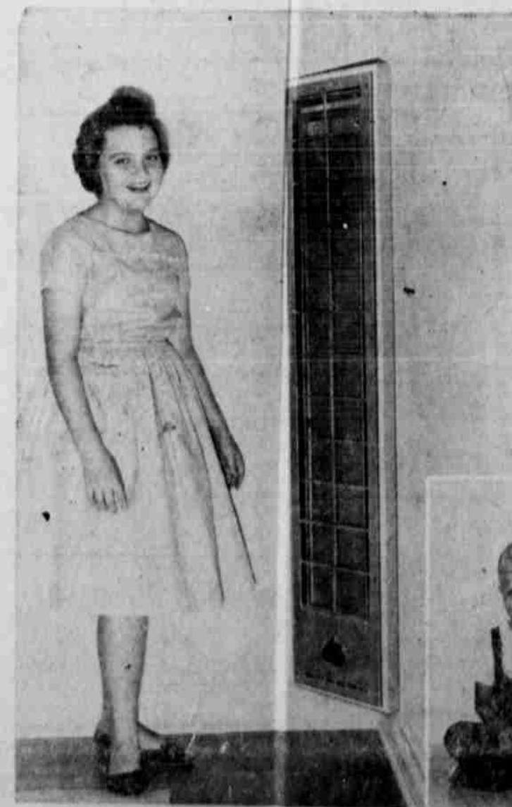
"Independent room control" is feature of electric heating system at H. H. Miller farm, Dawn, Texas. Radiant glass panels make attractive and safe installation and give exact degree of heating desired.
