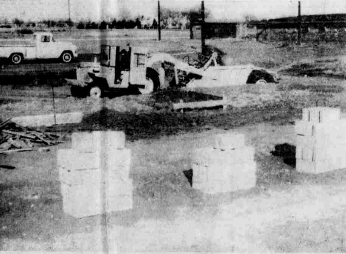
CONSTRUCTION IS UNDER WAY on a new privately operated public swimming pool here, located in Crescent Park just west of Crescent Park Motel. The pool, being built by Buck Oldham and Ace Bridwell, owners of the motel, is scheduled to be completed in time for the summer swimming season. The owners announced earlier this year that the pool would be about 60 by 150 feet, complete with filter system, heating unit, modern shower and dressing rooms and a concession stand. (STAFF PHOTO)
