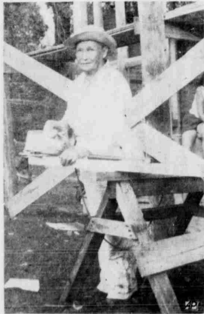
NEED HOUSE REPAIRED? SEE "MAMA"—"Mama" otherwise known as Mrs. Bils Davis Herrin is shown at work cutting rafters for her sons house at Kirbyville. "Mama" who is 71 has been carpentering for more than 50 years. (AP PHOTO)
