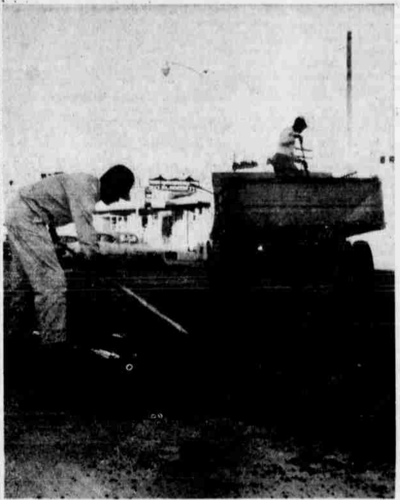
PATCHWORK —Thomson Construction Co. workers filled in joints in Littlefield's three concrete streets Monday, in an effort to take some of the bumpiness out of them. Worker James Jowers, in foreground, spreads a hot mix over a joint on Phelps Avenue after the mix had been thrown on the pavement from the truck in the background. XIT Drive and Littlefield Drive got the same kind of treatment. (STAFF PHOTO)
