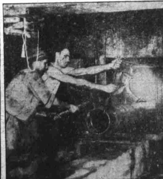
Cunning calculations of subterranean "navigators" brought directly together the two borings of a new vehicular tunnel 20 feet below the bed of the Hudson river. Sandhogs here are shown driving the survey pipe through to the tunnel started from the other side of the river—the first connecting link. The Midtown tunnel, a $37,000,000 PWA project, was progressing two months ahead of schedule. (Associated Press Photo)
