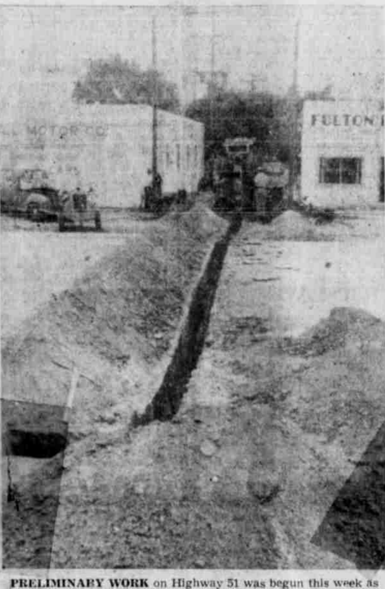
PRELIMINARY WORK on Highway 51 was begun this week as workmen dug down to water and gas lines under the highway. The lines must be lowered before widening improvements can start. Widening of the highway will begin as soon as this work is completed. It is expected to take another week.
