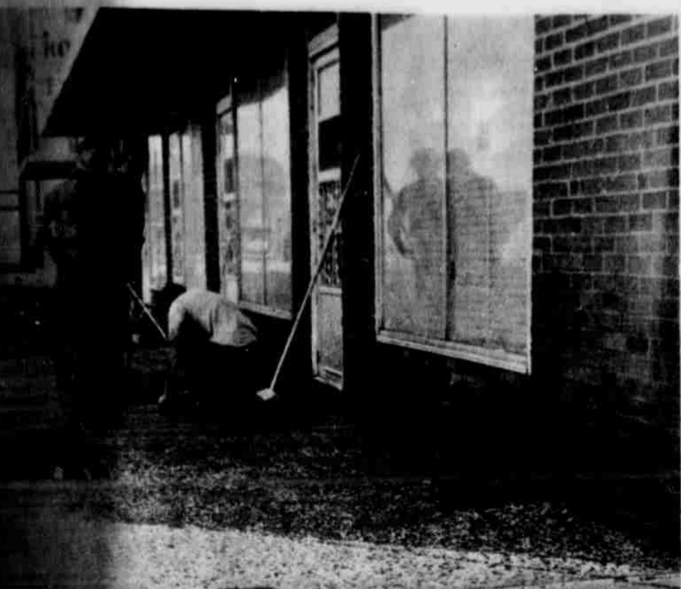
FIRST OF THE AGGREGATE -- The Shop downtown improvement project closer to completion each day as a part of the project is included. Shown is the first of the color aggregate being laid on Fourth between Phelps Ave. and LFD Drive. The contractors were setting the forms for the aggregate on Phelps yesterday and hope to pour today.
