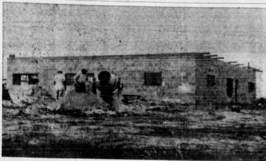
FIELDHOUSE NEARS COMPLETION —Scheduled to be completed three weeks from today, Littlefield High School's brand-new $18,000 fieldhouse will provide Wildcat athletes with the latest training facilities. The building is being constructed at a practice field just south of Highway 54. The practice field will be converted into the Wildcats' regular playing site in time for the 1957 football season.
