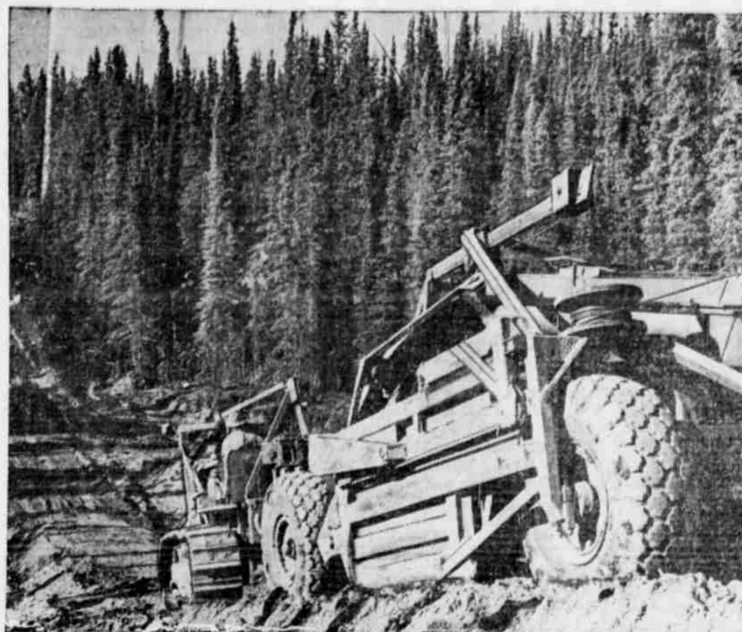
On this carry-all tons of earth are moved from a high section to fill in a low section of the Canada-Alaska Highway. Hidden two or three feet under the muskeg in some sections are glacial ice formations thousands of years old. When the muskeg is removed the ice melts, creating heavy morass, but the U. S. Army engineers have found a solution to the problem.
