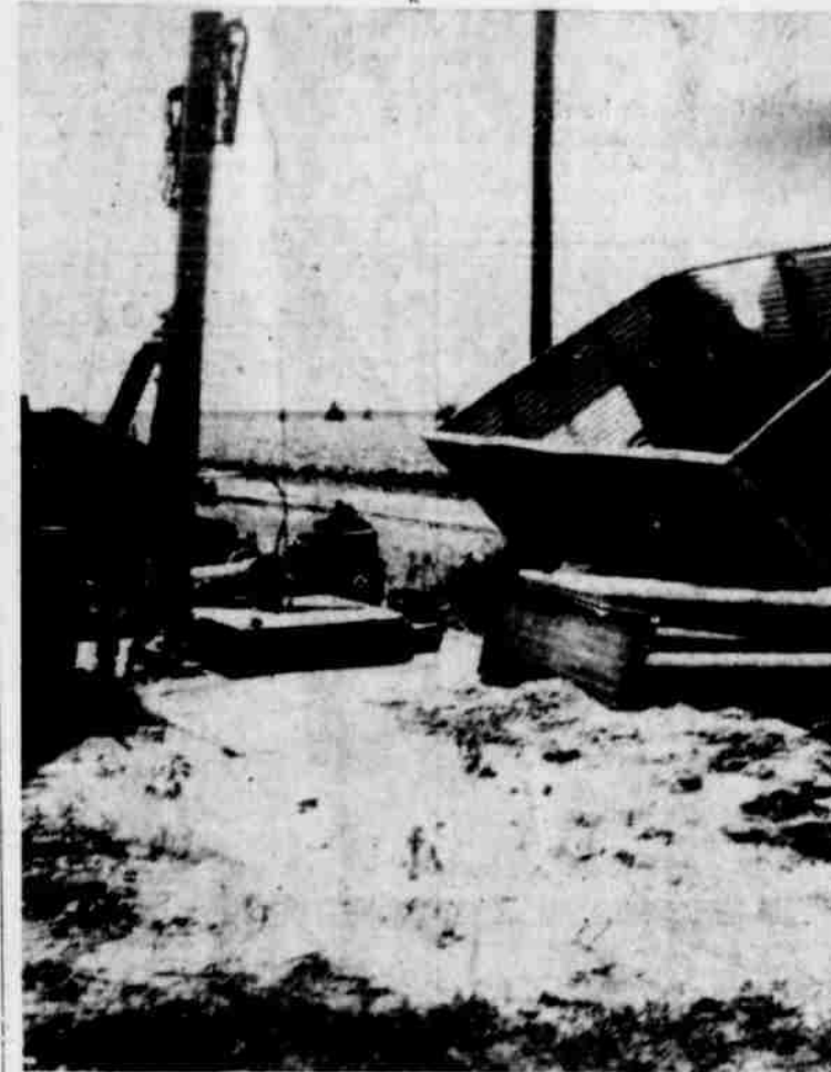
CITY WELL NUMBER SIX might well have a question mark hanging over it as city officials ponder whether or not repairs now going on will make a producer out of the well which went out early this week. The well is being worked over and it is hoped it will again be one of the big water producers for a town sorely in need of more domestic water. (Staff Photo)
