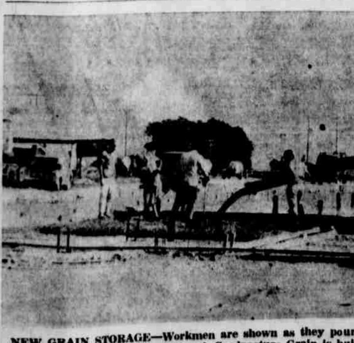
NEW GRAIN STORAGE—Workers are shown as they pour forms for a new grain storage bin located on the Lubbock highway north of the railroad. Goodpasture Grain is building the building and workmen estimated that the building will store 1,200,000 bushels of grain. Completion date will be some time in June.
