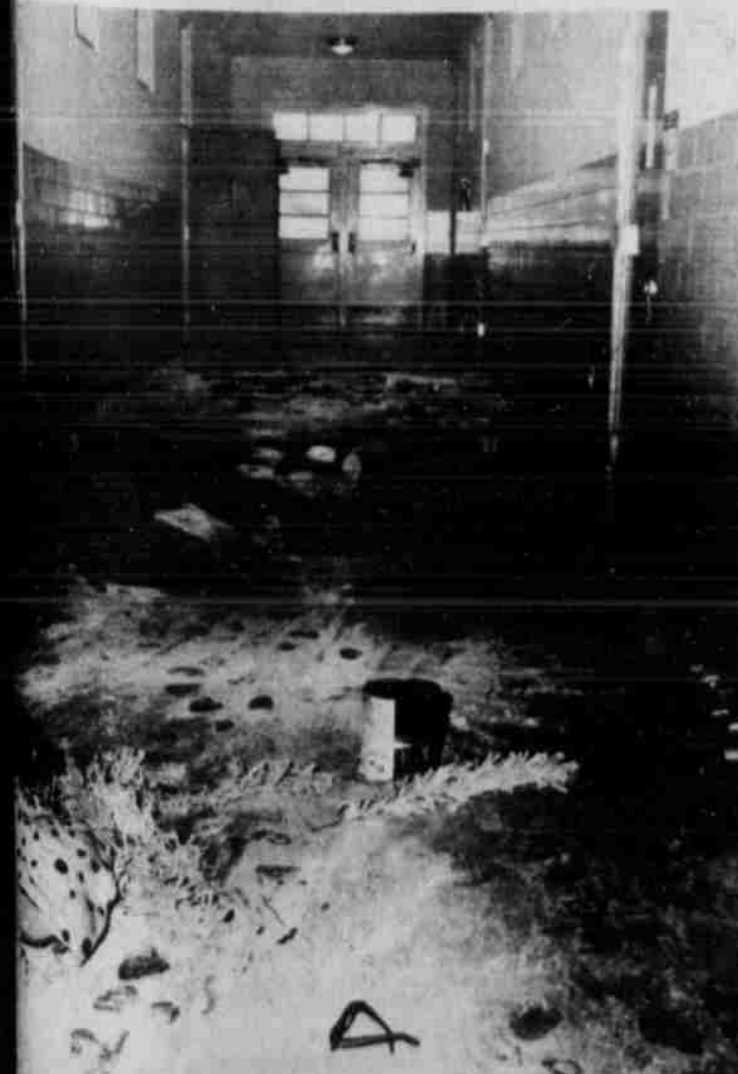
ESTIMATED DAMAGES in the vandalism of the Elementary I building amount to $2,000 to $5,000. This view of the south wing shows a portion of the damage to the building. Glass breakage and equipment damage losses are estimated to be high.
