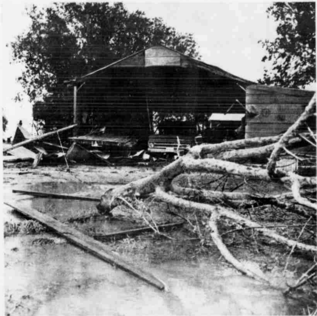
A BARN WAS DAMAGED considerably when the west end was blown out. A trailer, just inside the damaged end, had been loaded with 4,000 feet of aluminum pipe before it was blown 50 yards to the north and sucked inside. In the foreground is one of Fisher's prized fruit trees.
