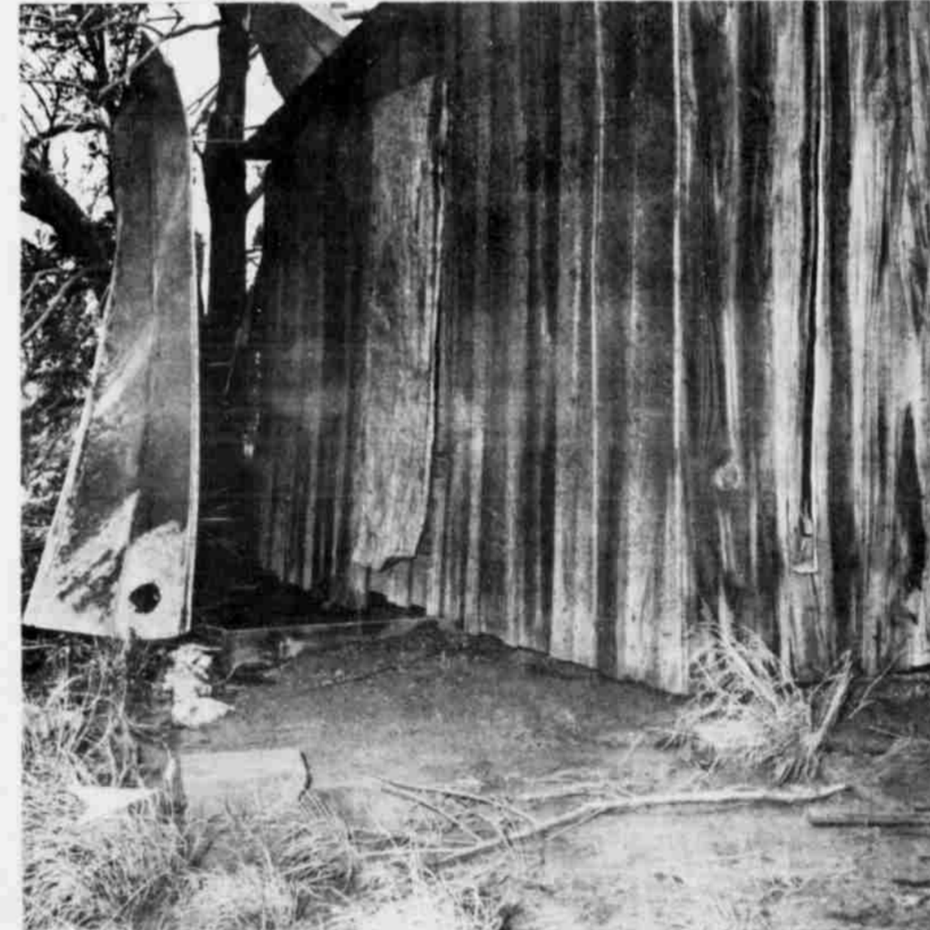
THE FOUNDATION of another barn was exposed when the building was moved about six feet to the north. The white arrow indicates the southeast cornerstone of the foundation.
