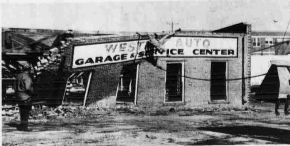
THE WALLS came tumbling down on the old garage building at the corner of XIT Drive and West Fourth Street this week. A new Goodyear Tire & Rubber retail store will be built at the location, with customer parking space to the east.
