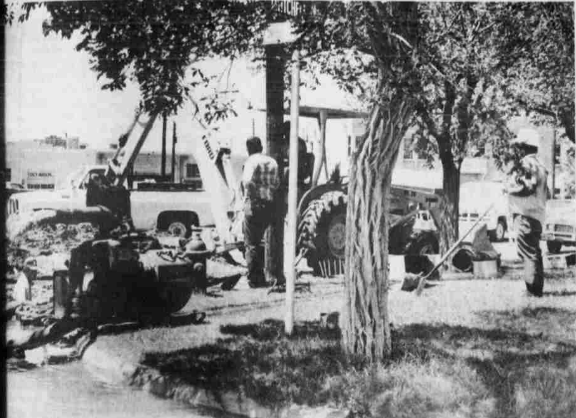
A BROKEN WATER main line on E. 5th flooded part of town and resulted in water having to be cut off for several hours Tuesday afternoon while city crewmen repaired the broken line. Beauty shops, restaurants and home owners alike felt the inconvenience of the water cutoff. (Staff Photo)
