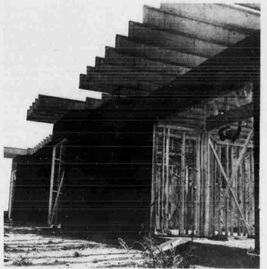
OFFICE CONSTRUCTION is getting well underway at the American Cotton Growers' Textile Plant east of town. Looking through the front of the building which faces east, a carpenter was caught in action Tuesday afternoon, as rafters and other bracing is nailed in place. Roofing will soon go on. (Staff Photo)
