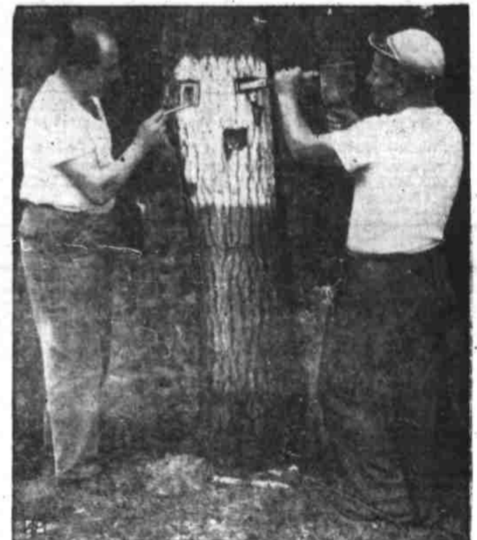
LIVE TREES — Workmen dig into tree trunk in British sector street, West Berlin, disclosing bark-covered dynamite charges set near end of last war to cause roadblocks.
