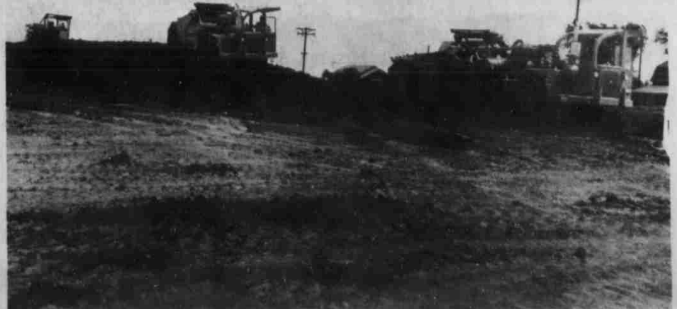
HEAVY EQUIPMENT is still on the job at the site of the new $30 million American Cotton Growers' denim mill east of Littlefield and dirt work is expected to continue
