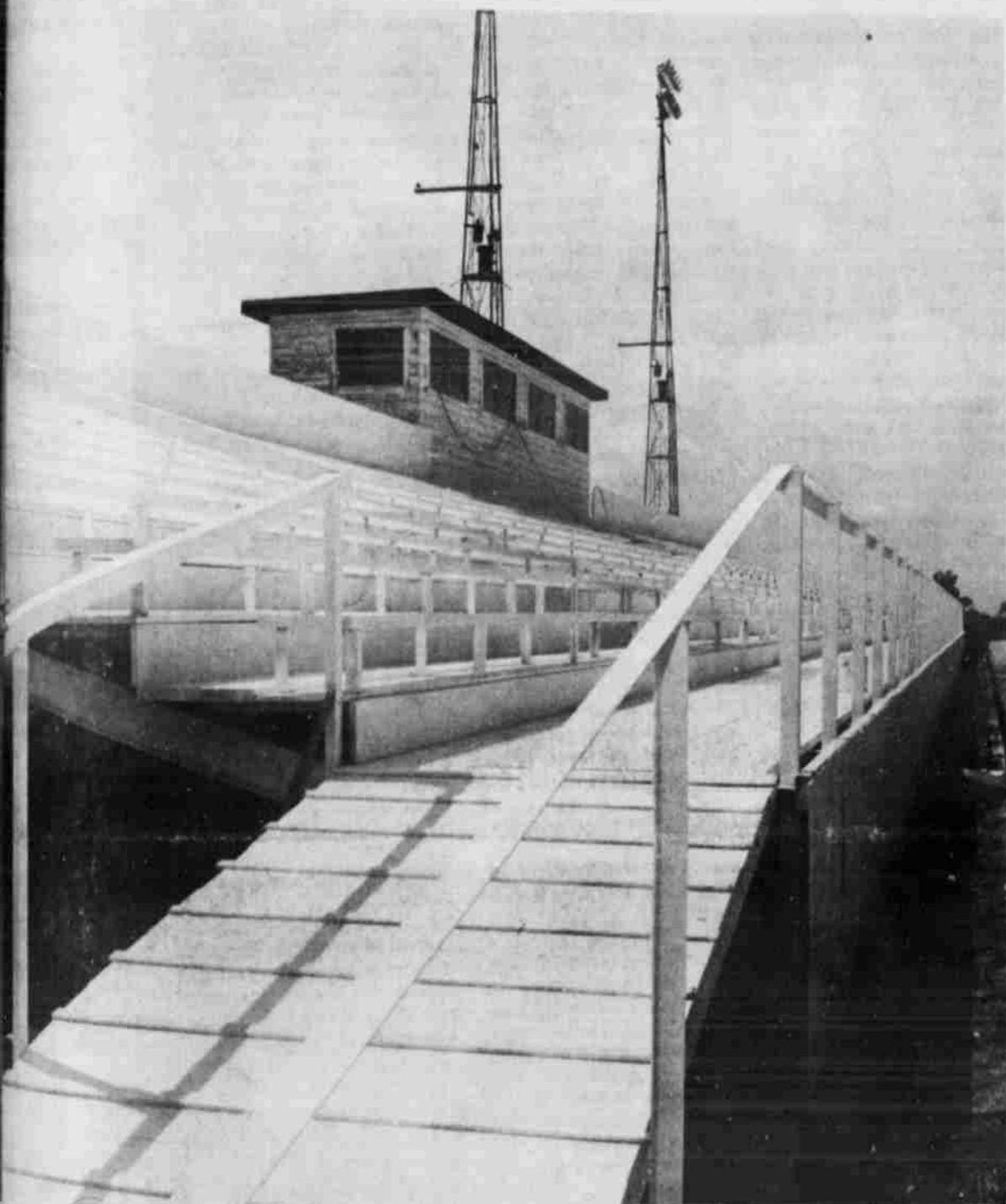
WORK IS NEARING COMPLETION on the visitors' bleachers at Wildcat Stadium, as the only thing lacking is final paint job. All the lumber in the old stands was
