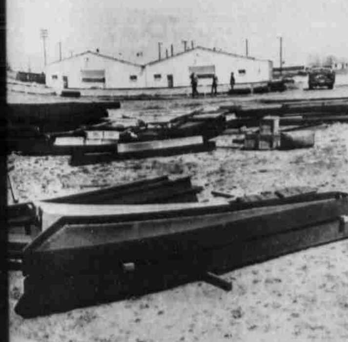
CONSTRUCTION of the foundation of the new Lamb County Ag Center has begun. The flooring will be poured in cement as soon as plumbing is complete. Ditches for the outer foundation have been dug, and cement forms are in place. (Staff Photo)
