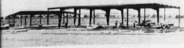
New Armes Equipment building being constructed on the by-pass of Littlefield on U.S. 84.
