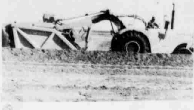
BENCH LEVELING on 23 acres of E. C. Curtis farm five and one half miles north of Springlake is in 50-foot strips from border to border. A pipe in the middle allows watering from both directions. The cut and fill was made with a scraper and maintainer. The strips are level from side to side with a .3 grade the length of the border and a six-inch cut and six-inch fill on each border. (SCS Photo)
