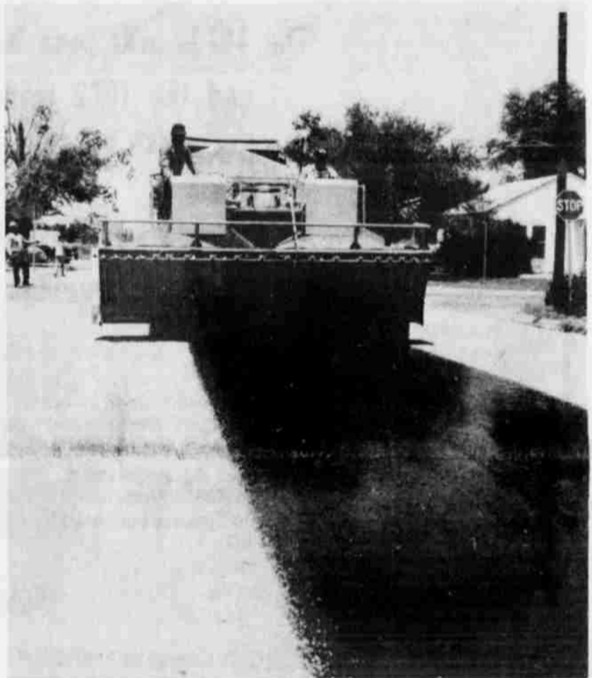
CONTRACTORS began seal coating some Littlefield streets early this week, and the project is calling for the repair of approximately 105,000 square yards of territory. Here, a gravel spreader covers the center of the street where the sealer has been sprayed. (Staff photo)
