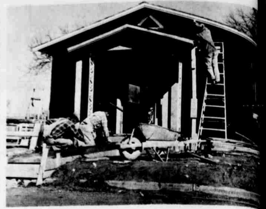
A NEW CHURCH BUILDING is being constructed at the corner of Hall Avenue for a Church of Christ congregation. Workmen who are laying the cement on the new sidewalk are, left to right, Cecil Gibson and Vernley. On the ladder is Y. C. Holmes, who is painting the wooden finish.
