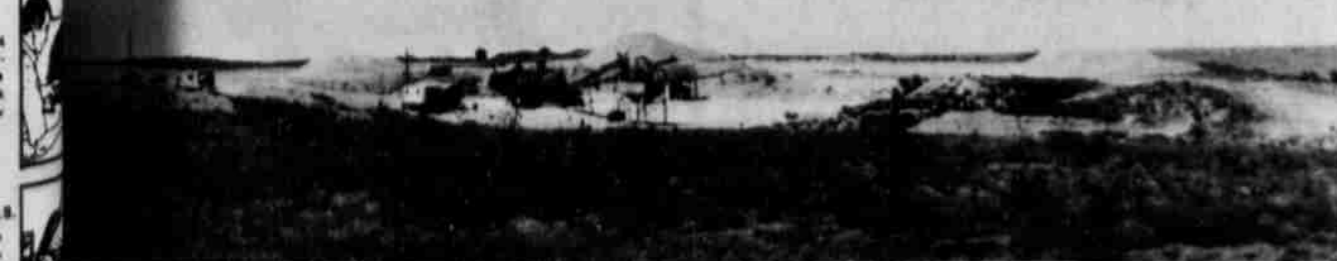
THIS ROCK crushing operation overlooks Bull Lake. Bill Perry, superintendent of crushers for Pioneer Pavers, Inc., heads the business which is located on part of the Badger estate. The lake below the work site lures the younger workers down for an occasional swim.
