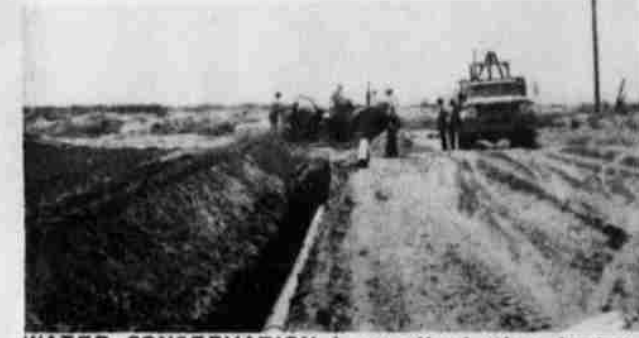
WATER CONSERVATION is practiced when buried irrigation pipelines are used instead of open ditches. Pipelines can deliver up to one-third more water to thirsty crops. Seepage from open ditches is eliminated. Above picture taken on Danny Bussanmus farm, northwest of Rocky Ford. (SCS Photograph)
