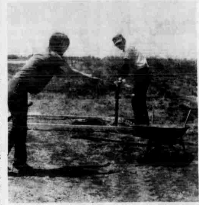
LORI AND JERRY Roberts are shown preparing for the new sign at the entrance of Bull Lake in the upper photo, and the completed project "The City of Littlefield Welcomes You To Bull Lake" is in the bottom photo. The new entrance is about a mile west of the old entrance and the roads have been graded and covered with caliche.
