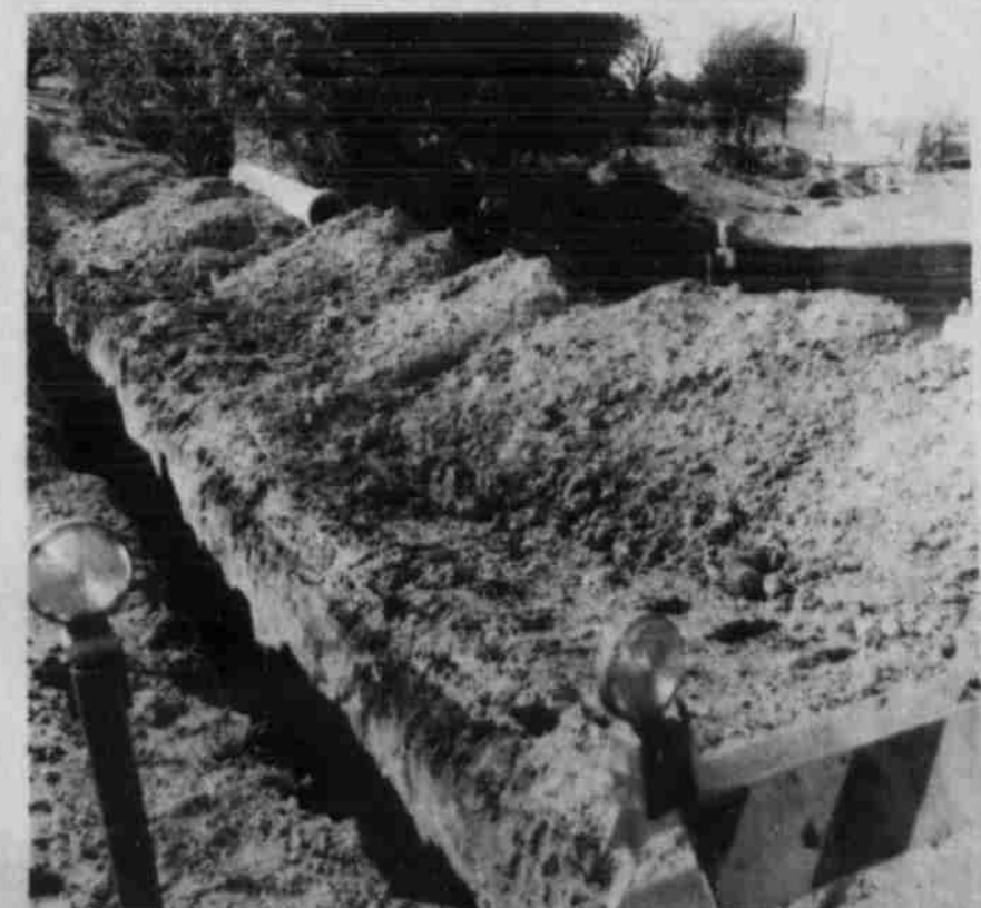
A 12-INCH WATER LINE will come down this ditch and be connected westward with the line which goes underneath the highway (shown in front of the parked vehicles in the right background) and toward the new textile plant now being constructed east of Littlefield. Alongside the road ditch is hardware for connections. (Staff Photo)
