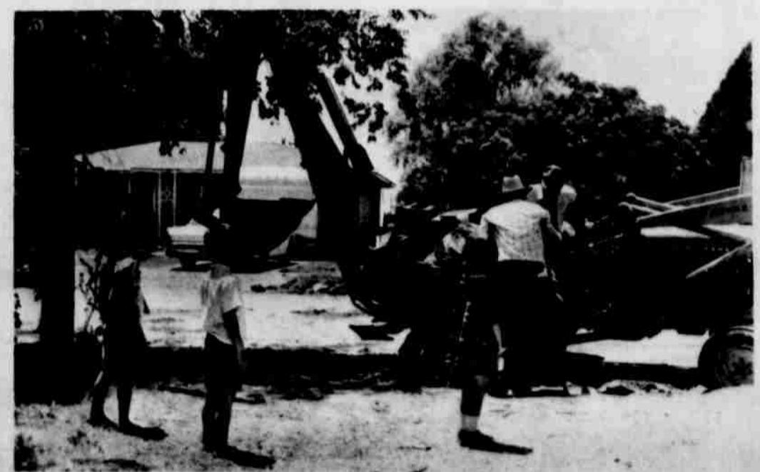
SIDEWALK SUPERINTENDENTS are more plentiful than construction workers on South Phelps where the street is being widened and raised. Watching two employees who were tearing out the curbs Tuesday are Robert and Michael Lewis Austin, left, and Vivian Diane Cooper and Bill Cooper.
