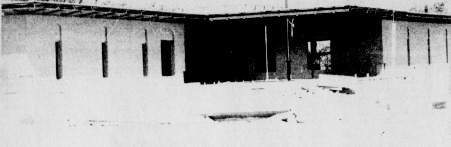
BANK BUILDING GOING UP . . . . . The new location of Muleshoe State Bank is beginning to look like a building now since the walls have been erected on the building. Construction seems to be progressing smoothly at the present time. The new larger building to house the Muleshoe State Bank is scheduled to be completed by early fall this year, barring any complications.
