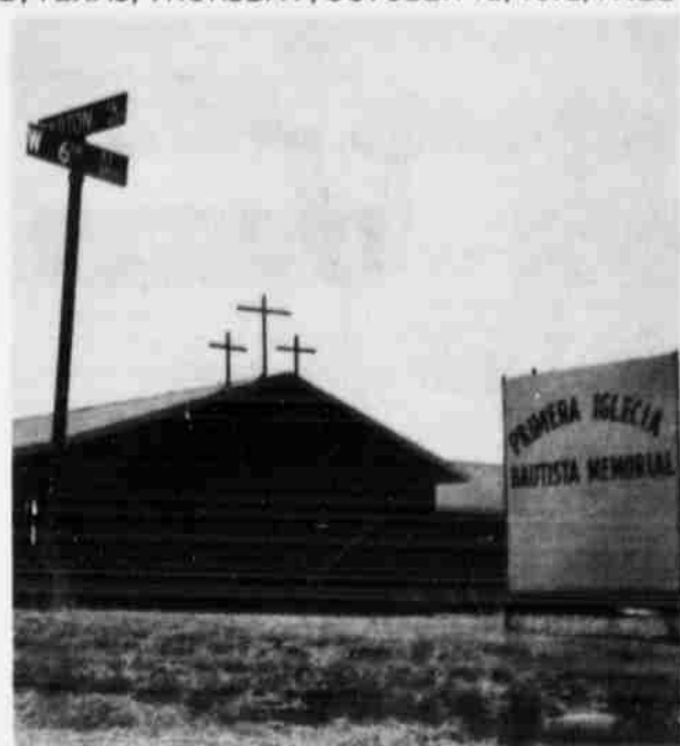
CONSTRUCTION continues at Primera Iglesia Bautista Memorial, located at West Sixth and Barton Streets in Littlefield. Three crosses now accent the skyline of the new educational unit which is being built by members of the church. (Staff Photo)
