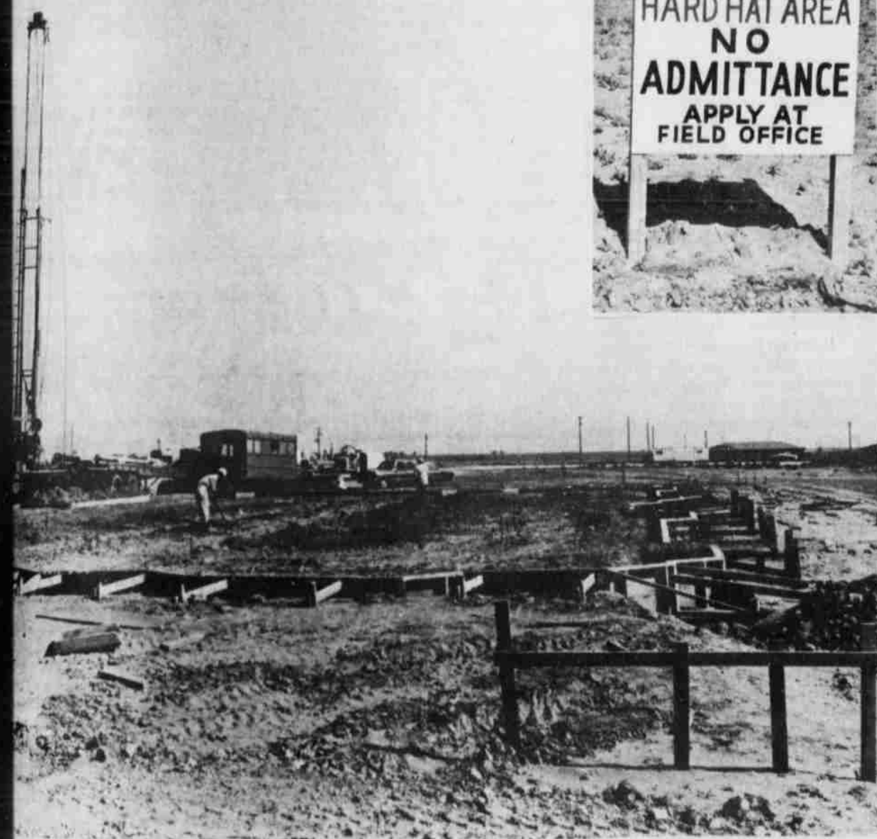
MENT FRAMES for a portion of the Denim Textile floor are in place, and workers continue operations before the floor is poured. Heavy machinery continued to work nearby, preparing the larger portion of
