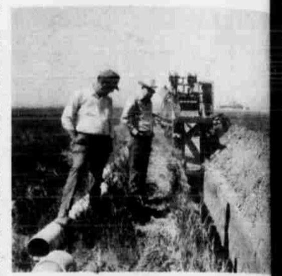
PIPELINE FOR a high pressure underground system four circular sprinklers was drilled 10 miles west of Littlefield at the edge of the sandhills. Wayne R. and Gil Webster are shown here watching the progress of the ditching. White and H. L. Cain bought the farm year. SCS personnel remind farmers that there is money available for pipelines and other conservation practices through the REAP program. (SCS Photo)
